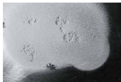
Rust pitting must be sand-blasted before the prepared area is ready for further treatment.
